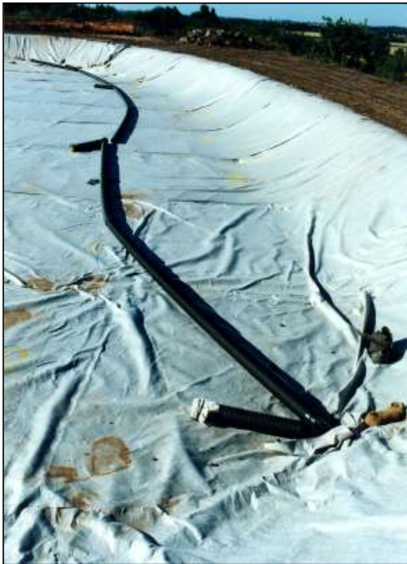
View shows the protective blanket of geotextile laid over the HDPE membrane, before the stone is placed
